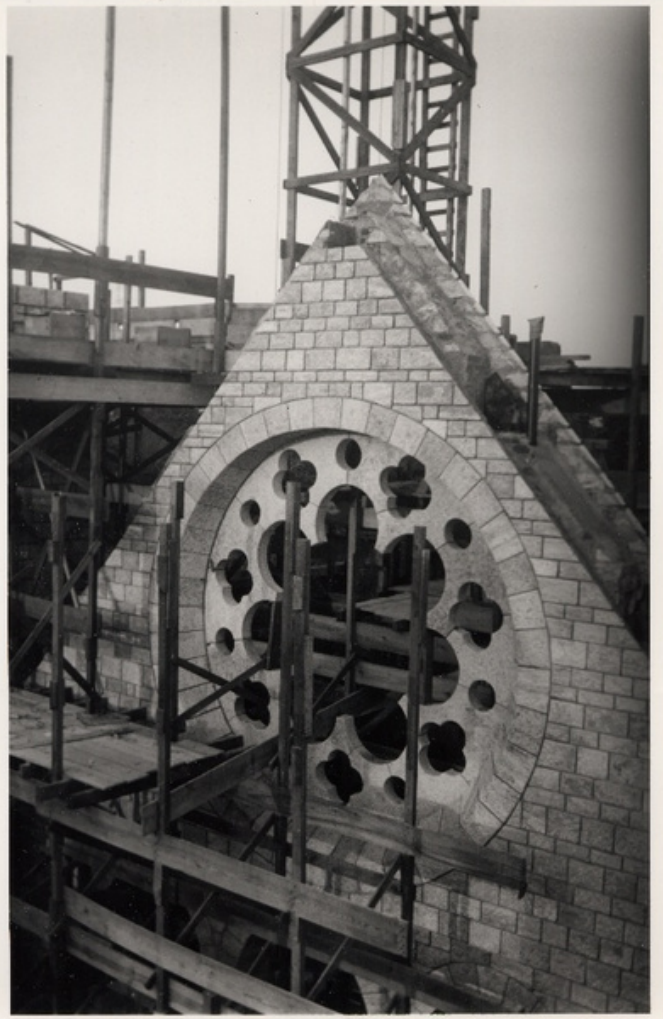
The construction of Glencairn's Great Hall in the 1930s. The tracery for the rose window was built but the window had not been installed yet.
